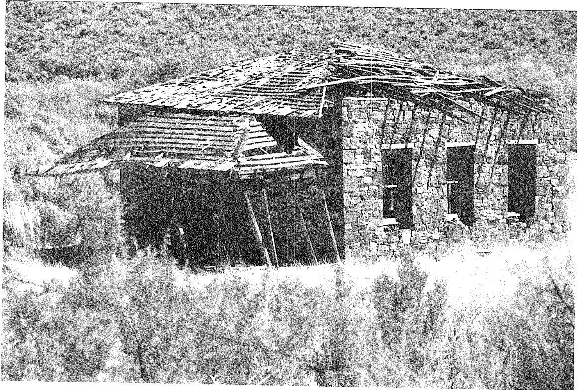
School Building on Trout Creek Located about 3 Miles West of Defenbaugh Ranch on White Horse Ranch Lane
